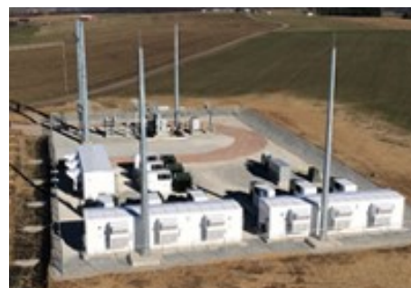
Myersdale PA Energy Storage | NextEra
